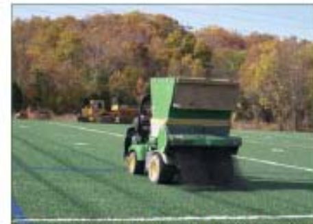
6. Field lines installed. Infill system consisting of cryogenic rubber sand and topsoil and groomed.
