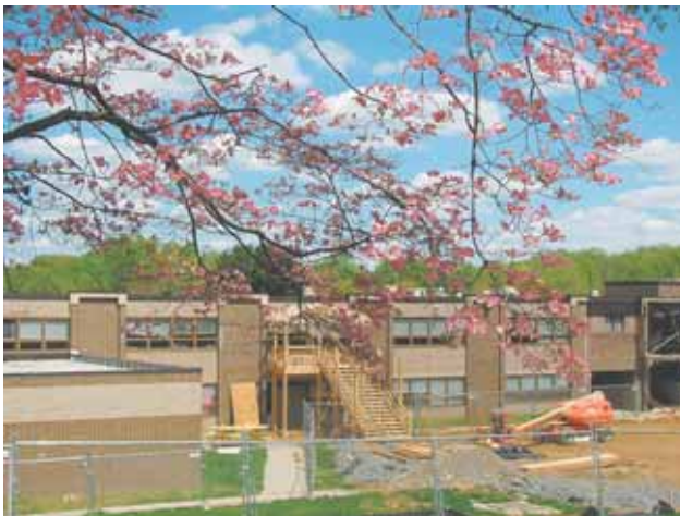
PHOTOS BY KEN MOORE/THE CONNECTION Langley High School is currently being renovated in a project approved by a bond referendum in 2013.
